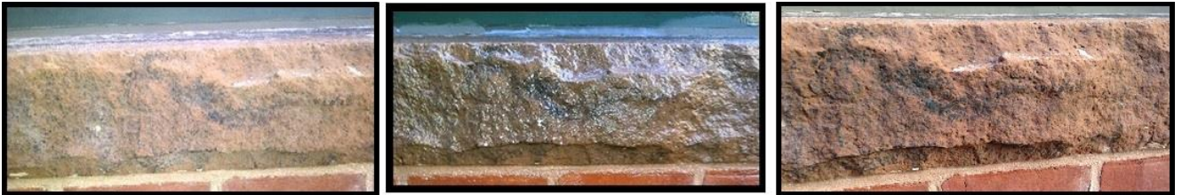
The brownstone window sill, before, during and after pressure washing [Left to Right] 137
