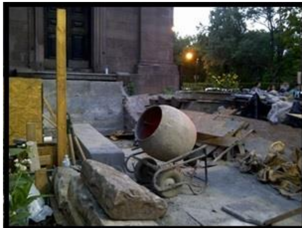
Arlington Church, the corner of Boylston and Arlington Street, Boston, MA. Brownstone has been removed to install handicap ramps, 2015. 39
