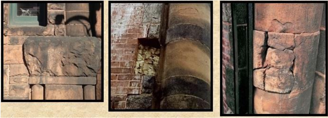
Repointing, missing piece of brownstone, and impact damage located on 951 Boylston Street, Boston, MA. [Photos Left to Right]
