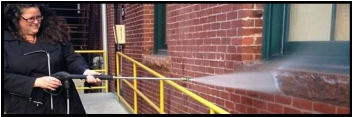
Patti Vaughn pressure washing the brownstone window sill, 951 Boylston Street, Boston, MA 136
