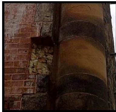
A missing piece of brownstone from 951 Boylston Street, Boston 118
