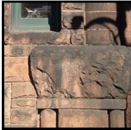
Mortar missing between the brownstone column pieces
